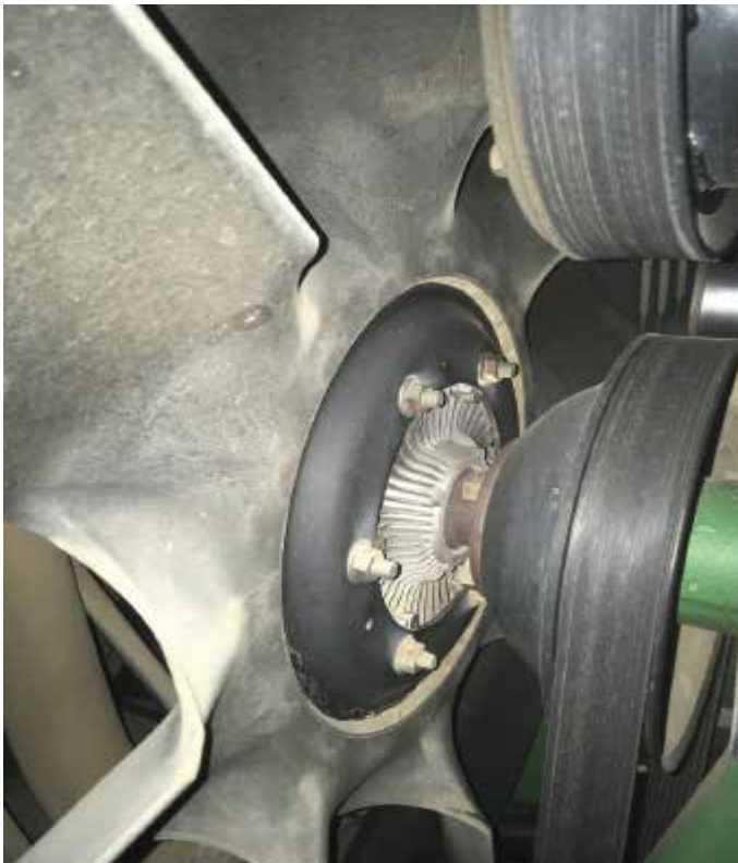
Check to ensure there is no play on the viscous drive hub on the engine cooling fan drive. Make sure, too, that the hub is operating properly.
