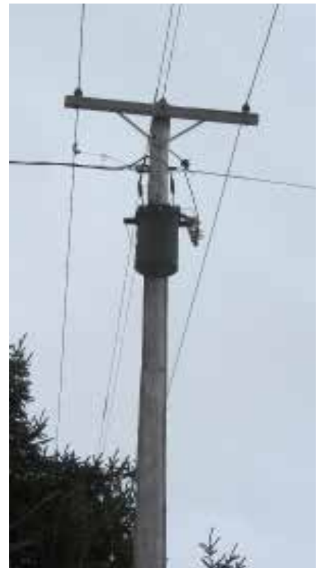
A typical farm single phase transformer.
