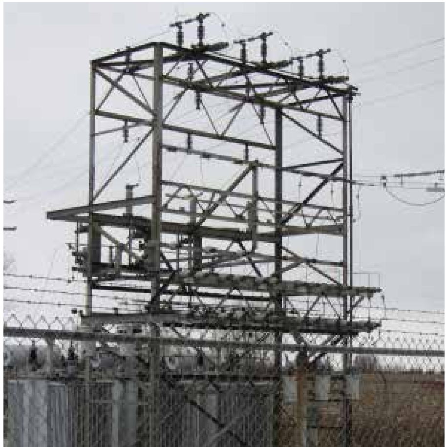
A local hydro distribution station reduces the voltage down from 27.6 kV to distribution voltage.
